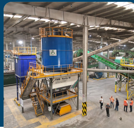
Mechanical Biological Treatment Plant
