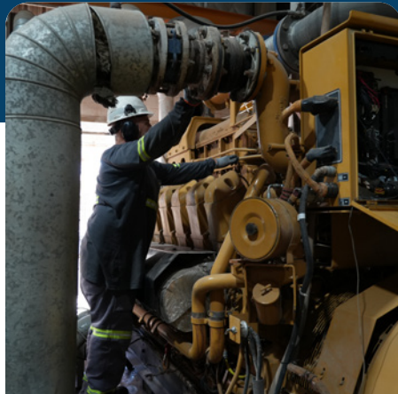
Gas Treatment and Energy Generation Plants
