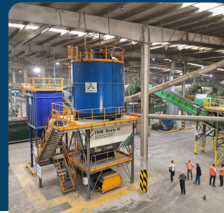
Mechanical Biological Treatment Plant
